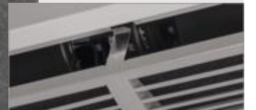
Air intake grille
