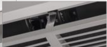
Air intake grille
