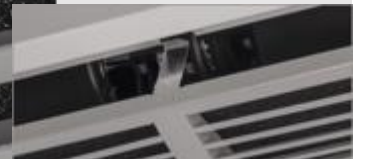
Air intake grille
