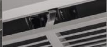
Air intake grille
