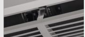
Air intake grille
